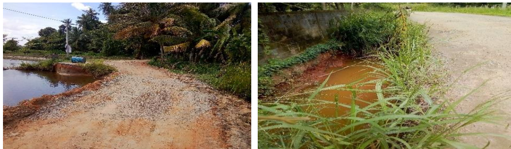
(PU-03 Road No. 17 from Badura to Sadanangama Katuwagoda Road via Maningala – Chanage 1+010) (PU-03 Road No. 38 Dickwela Road )
