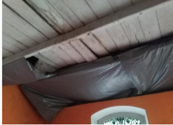
(Dilapidated Estate Bungalow in suduwelipotha Estate)
