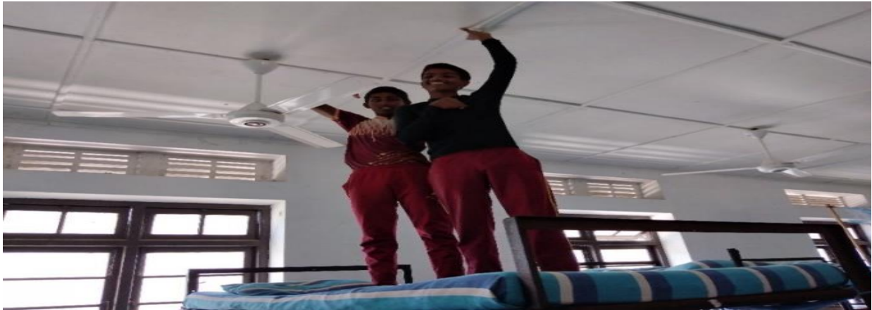
Insufficient gap between the upper bed and the ceiling
