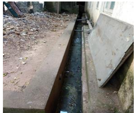
Unclean drain at the back of the kitchen
