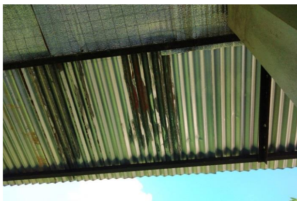
Roofing sheets had been corroded
